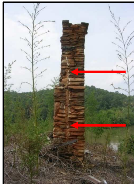
Figure 4: View of vertical joint shadow on south side of chimney (looking north)
