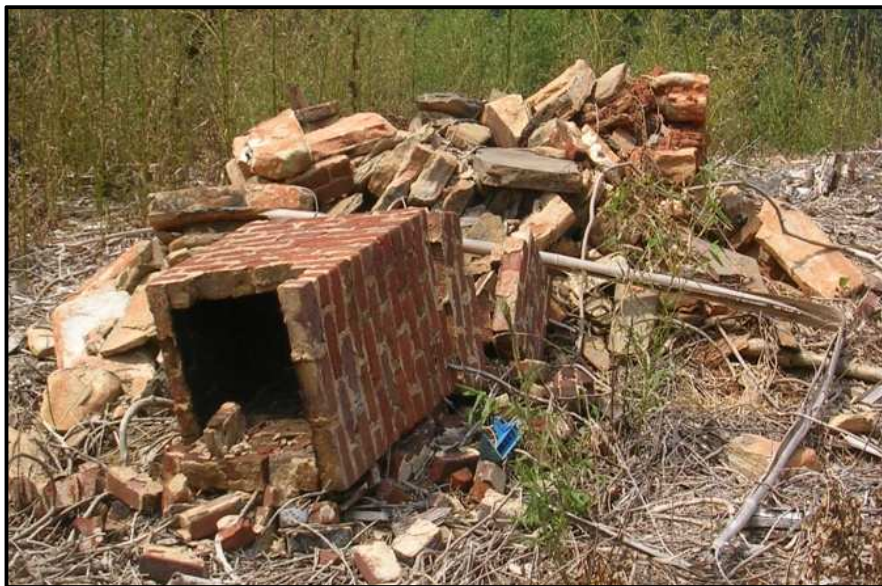
Figure 6: View of collapsed stone/brick chimney
